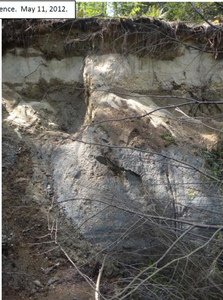
Figure 7. Field stop 26, photo 62 from Wilson Creek showcasing the landslide at the Bloom residence (Horel, 2012).
